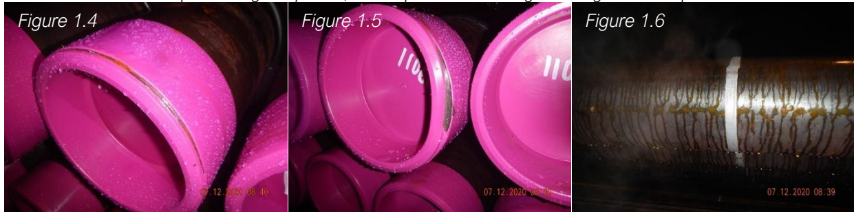
Figure 1.4 Figure 1.5 Figure 1.6 Damage to end caps – pipe join and steel condition
